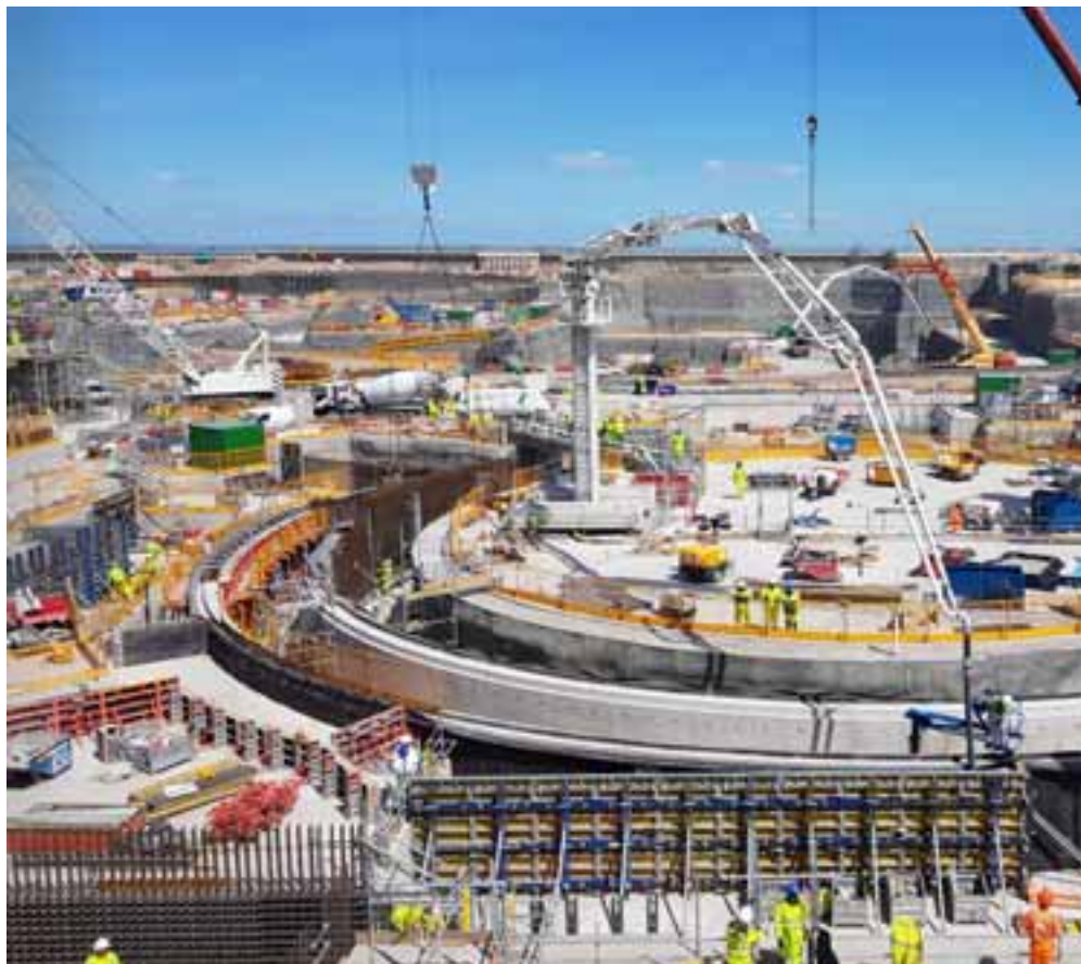
Work in progress at the new reactor site at Hinkley Point, Somerset. Photo EDF.
